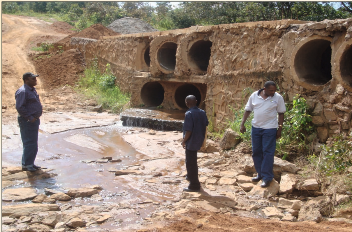
Figure 5.16: The audit team assessing the quality of works of a vented drift along Miangalua – Chombe – Kyamatundu Road in Sumbawanga District Council
