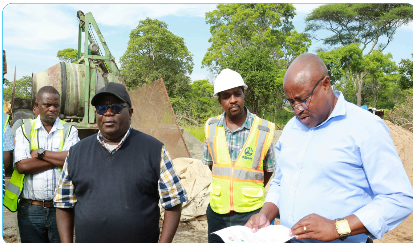
Deputy Minister of Works, Eng. Godfrey Kasekenya (left), inspects the road works in Katavi recently
